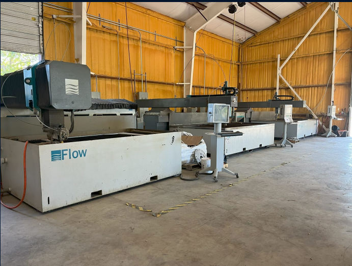
THREE WATERJETS INSTALLED AT THE ENTERPRISE LOCATION
